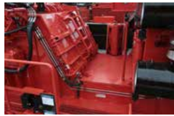
Extended Maintenance Platform
